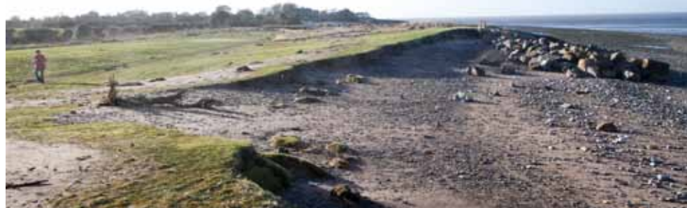
Sea defences exposed on Grune Point
